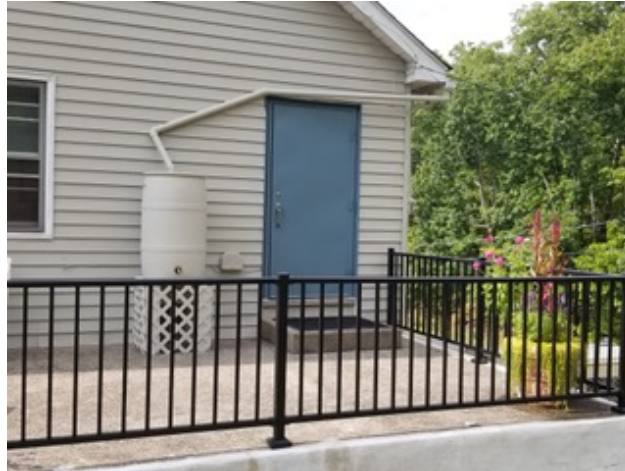
Tinicum Township's Public Works Department installed a rain barrel for the Tinicum Township Municipal Building.
